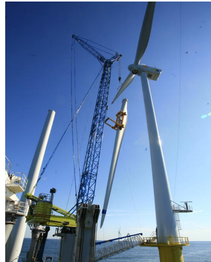
Precision is essential when the nacelle is placed in the right position
